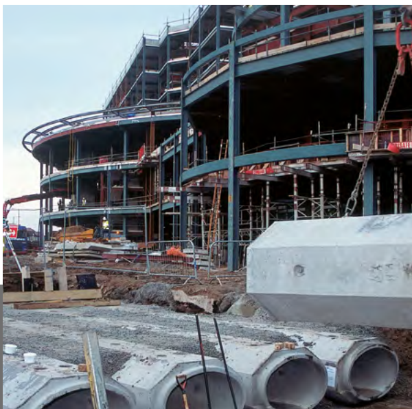
Elliptical tanks used for flood attenuation at Twickenham Rugby Stadium.
